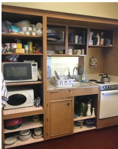
(Photo 48) Non-compliant staff break area
