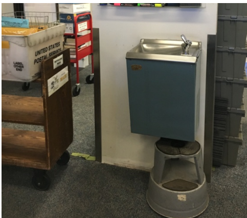
(Photo 08) Non-compliant Drinking Fountain
