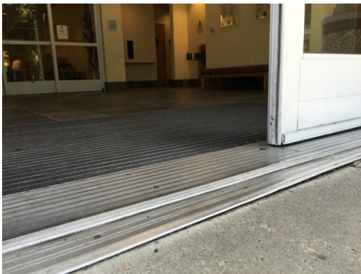
(Photo 51) Damaged threshold
