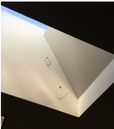
(Photo 69) Ceiling water damage
