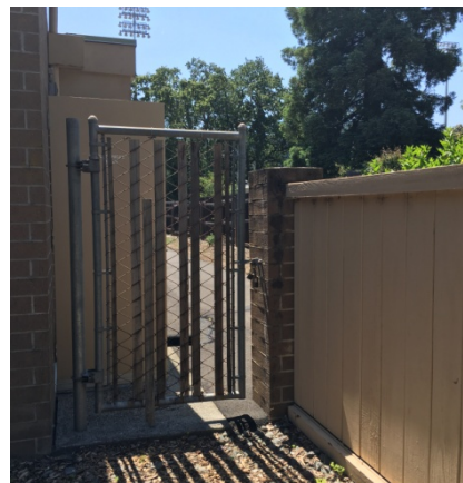
(Photo 91) Non-compliant path of travel
