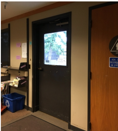
(Photo 32) Non-compliant egress door
