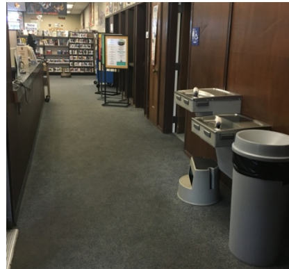
(Photo 25) Non-compliant pocketing along circ.
