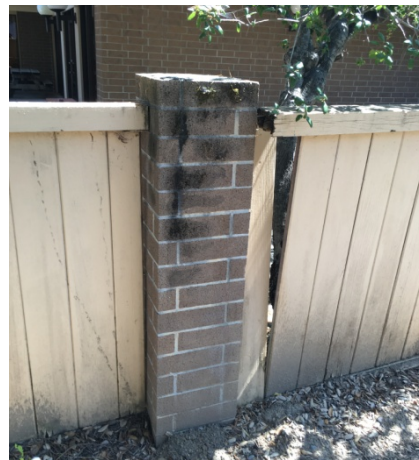
(Photo 85) Damaged perimeter fencing
