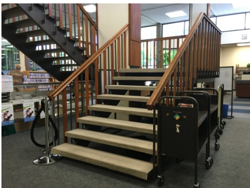
(Photo 10) Non-compliant handrail extensions & visual contrasting warnings
