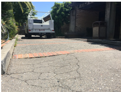
(Photo 62) Non-compliant path of travel
