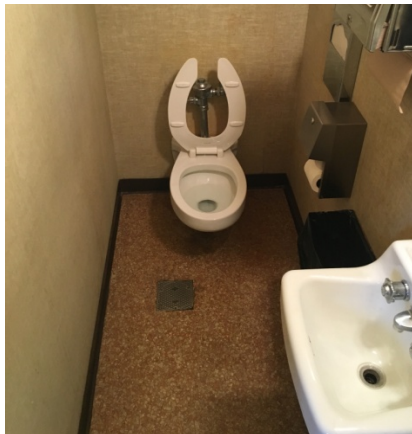
(Photo 26) Non-comp. restroom
