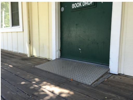
(Photo 74) Non-compliant threshold
