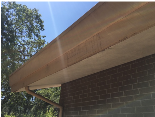
(Photo 84) Water damage to fascia boards
