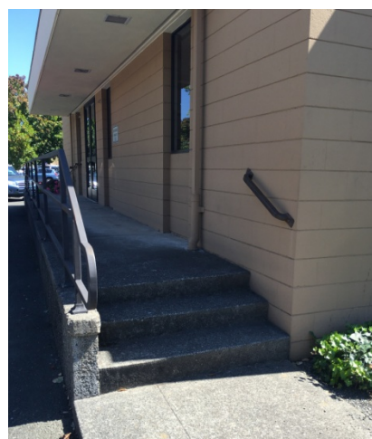
(Photo 16) Non-compliant stair to Annex
