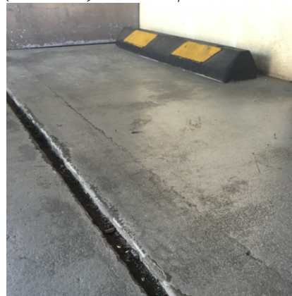
(Photo 11) Concrete gap @ Staff Entrance
