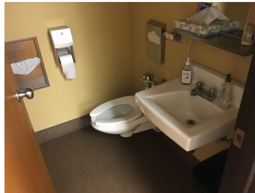
(Photo 89) Non-compliant staff restroom
