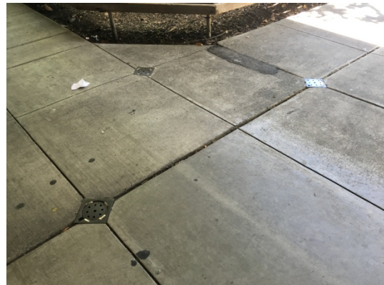
(Photo 03) Concrete pavement separation
