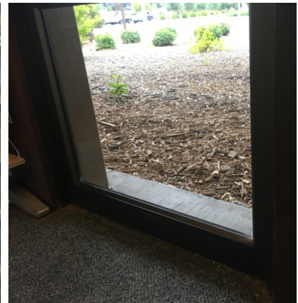
(Photo 28) Non-compliant exit
