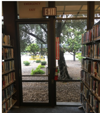
(Photo 27) Non-compliant exit
