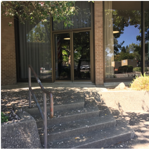
(Photo 06) Non-compliant Egress Stair
