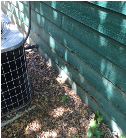
(Photo 77) Peeling paint @ base of wall
