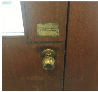
(Photo 47) Non-compliant door hardware
