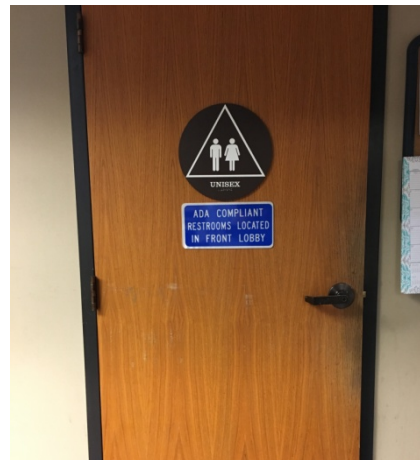
(Photo 33) Non-compliant staff restroom
