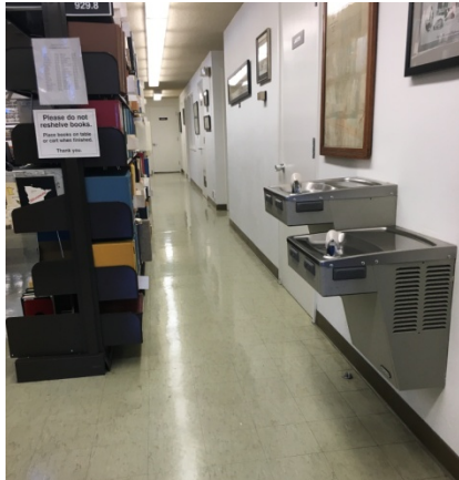
(Photo 17) Non-compliant high-low drinking fountain
