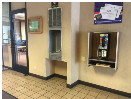
(Photo 63) Non-compliant drinking fountain
