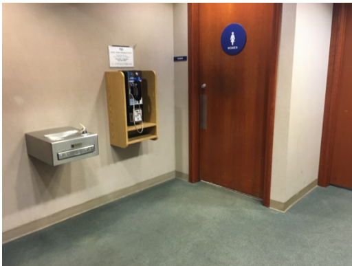
(Photo 67) Non-compliant drinking fountain
