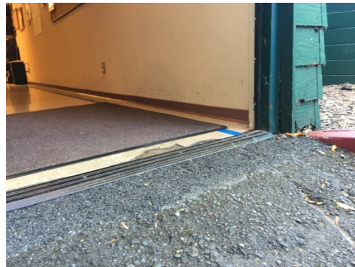
(Photo 78) Non-compliant path of travel
