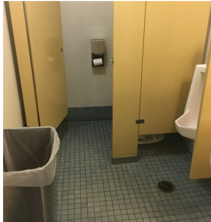
(Photo 18) Non-compliant men's restroom
