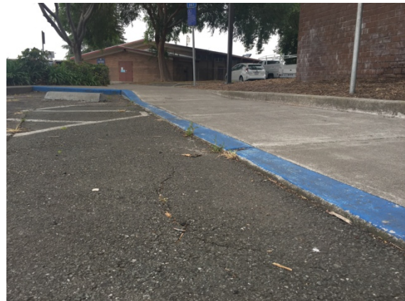
(Photo 41) Non-compliant accessible path
