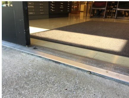
(Photo 22) Threshold requiring maintenance
