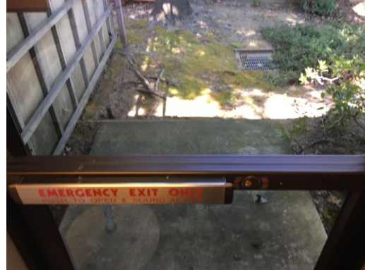
(Photo 65) Non-compliant path of travel
