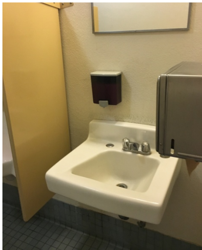
(Photo 19) Non-compliant vanity
