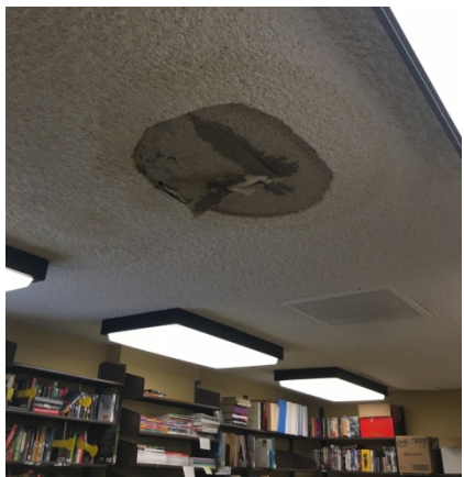
(Photo 90) Water damage to ceiling
