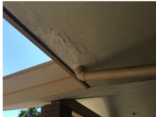
(Photo 83) Water damage to soffit
