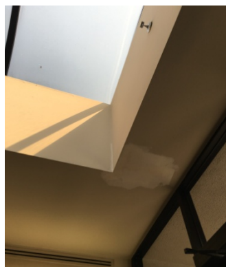
(Photo 70) Ceiling water damage
