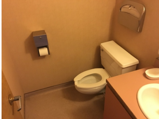
(Photo 64) Non-compliant staff restroom
