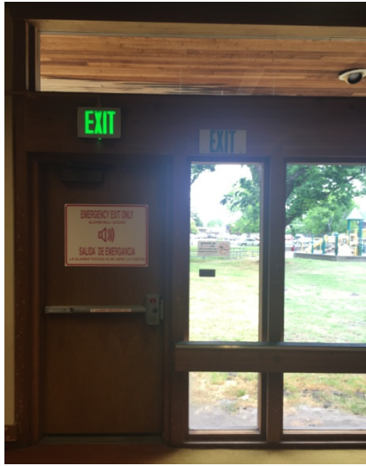
(Photo 44) Non-compliant path of egress
