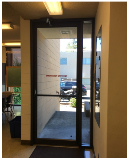
(Photo 20) Egress door w/o illuminated exit signage
