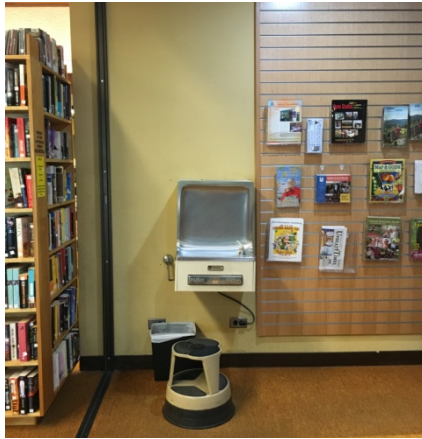
(Photo 86) Non-compliant drinking fountain
