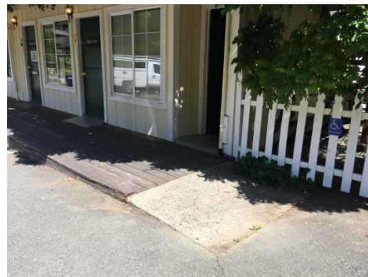
(Photo 73) Non-compliant path of travel
