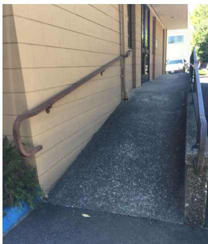
(Photo 15) Non-compliant ramp to Annex
