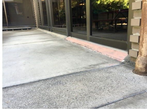
(Photo 07) Non-compliant Door Threshold
