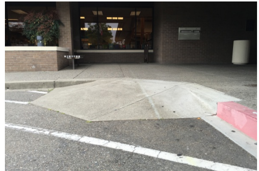
(Photo 31) Non-compliant path of travel
