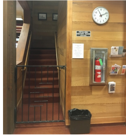
(Photo 45) Non-compliant public stair
