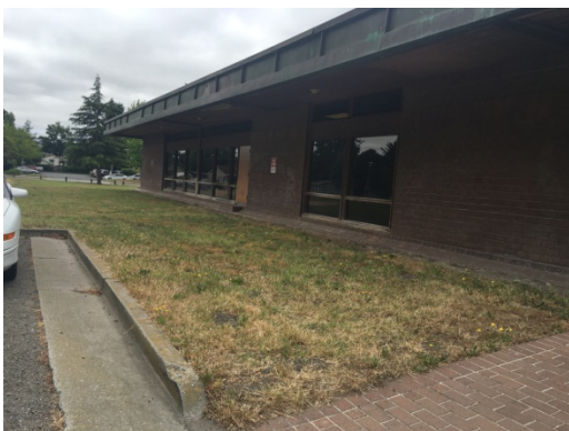
(Photo 42) Non-compliant ramp & threshold
